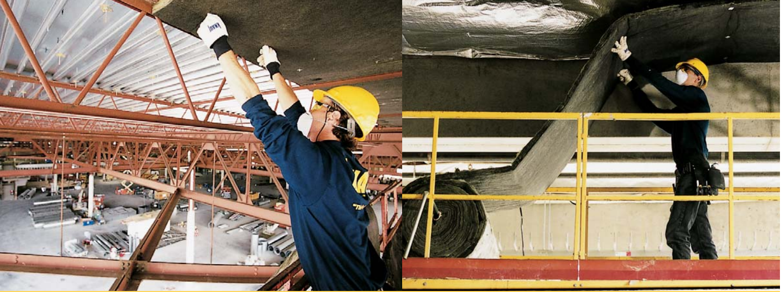
Knauf Wall and Ceiling Liner M was used in the Stadium Exhibition Center as a ceiling blackout treatment and for its thermal and acoustical benefits. In the Main Exhibit Hall (left), it was used under the metal roof deck primarily for sound control and aesthetics. In the “swing space” (right), it was used in combination with R-11 batt insulation and a foil vapor barrier to achieve the thermal envelope design requirements.
