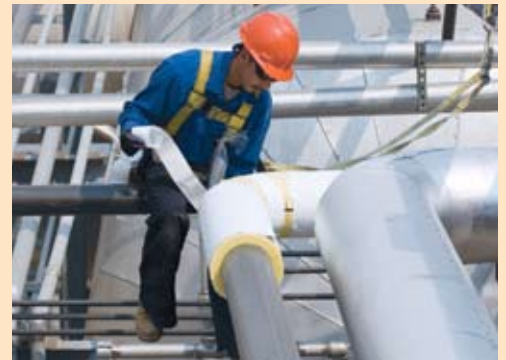
Installation of Knauf 1000° Pipe Insulation in the retrofit areas allowed for non-stop production of ethanol.
